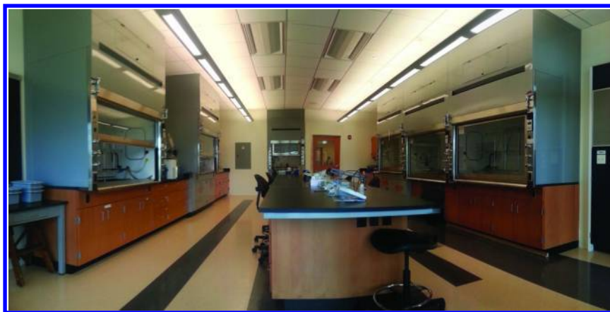
Figure 3. Panoramic photo of the HVAC intensive laboratory. (see color insert)
