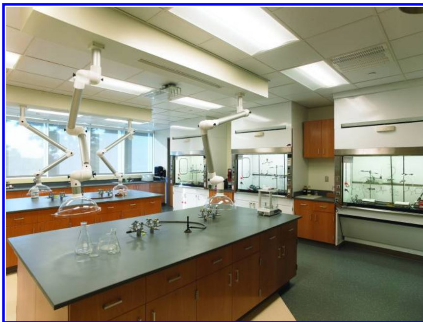
Figure 3. Fume extractors at Nazareth College are movable. (photo courtesy of Tim Wilkes Photography). (see color insert)
